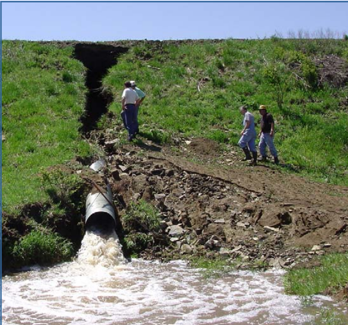
Internal erosion of a dam.
