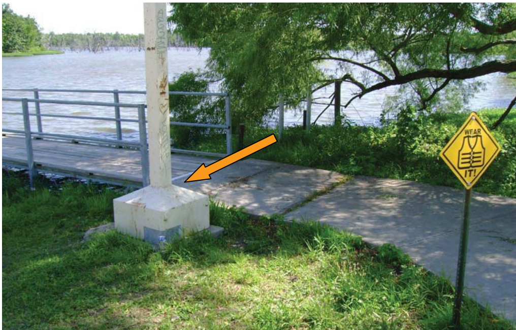
Figure 3b. Close-up view. Lake level was measured from the water surface to the top of the concrete dock anchor pad. (Arrow indicates specific location on pad).
