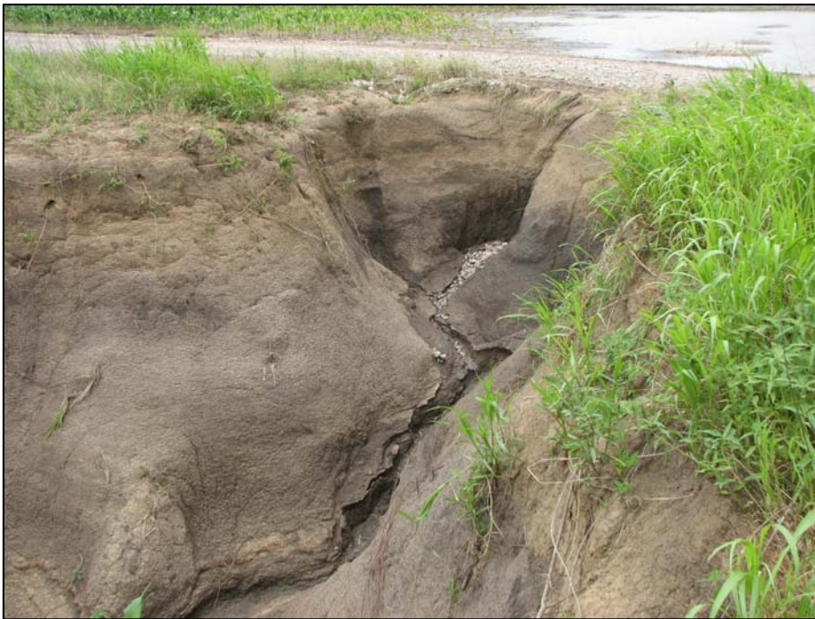
Figure 14. Gully erosion caused by road presence.
