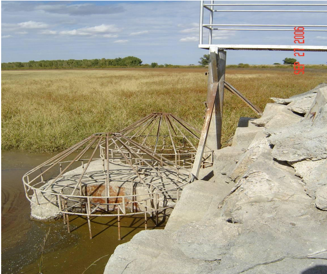
Old Outlet works with silt and grass indicating capacity loss in Lake McKinney
