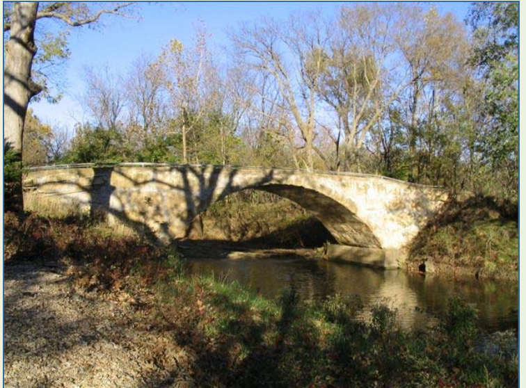
Stone bridge over Badger Creek, Cowley, County. Photo courtesy Kansas Geological Survey.
