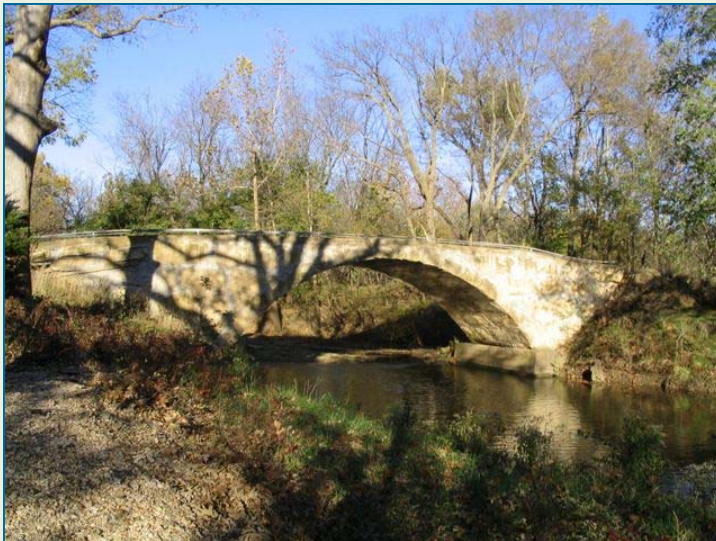
Stone Bridge over Badger Creek, Cowley County Photo courtesy Kansas Geological Survey
