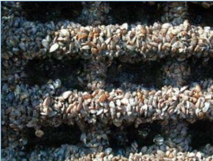
Zebra Mussel build up on wet well trash rack , El Dorado Lake
