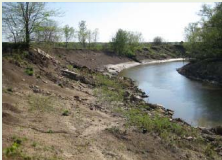
Figure 11. KAWS Level 1 Assessment of the Marmaton River - Photo of an unstable streambank on the Marmaton River
