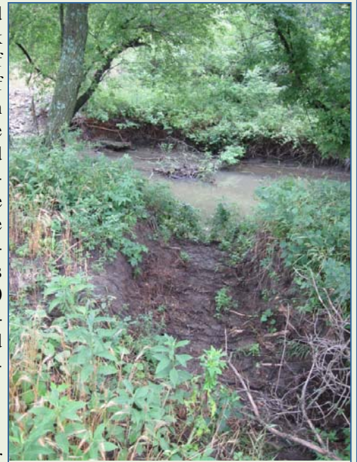
Figure 9. Gully Erosion on Dragoon Creek
