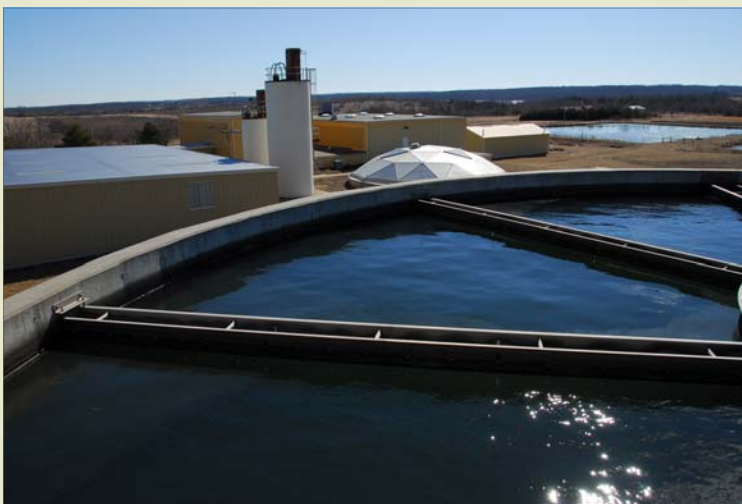
Tri-District Clarifier. Photo courtesy Dennis Schwartz
